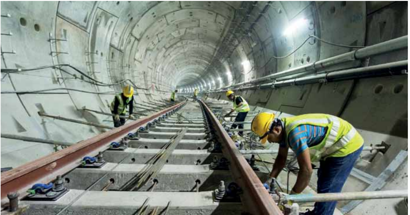
4 Klang Valley MRT Linie 1: Bauarbeiten in der Nähe des Pudu-Schachts Klang Valley MRT line 1: Execution of works in the tunnel close to Pudu shaft
