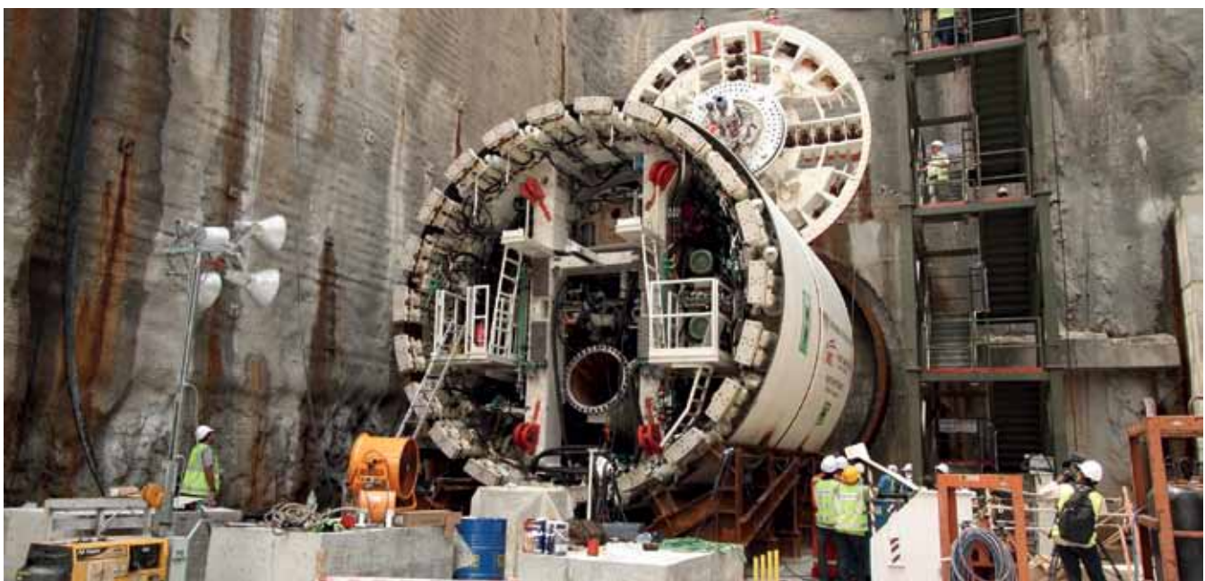
3 Klang Valley MRT Linie 1: Montage einer VD-TBM im Startschacht Cochrane Klang Valley MRT Line 1: Assembly of the VD TBM at the Cochrane launch shaft
